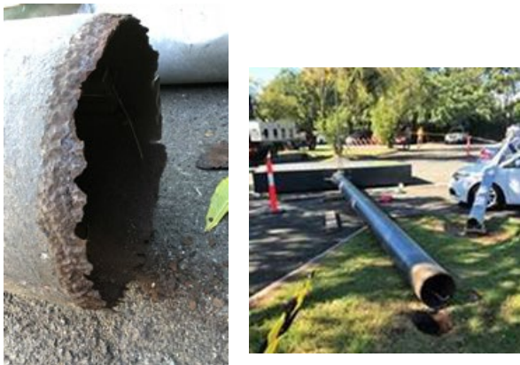
Failure area at the base of the support post. Collapsed sign.
